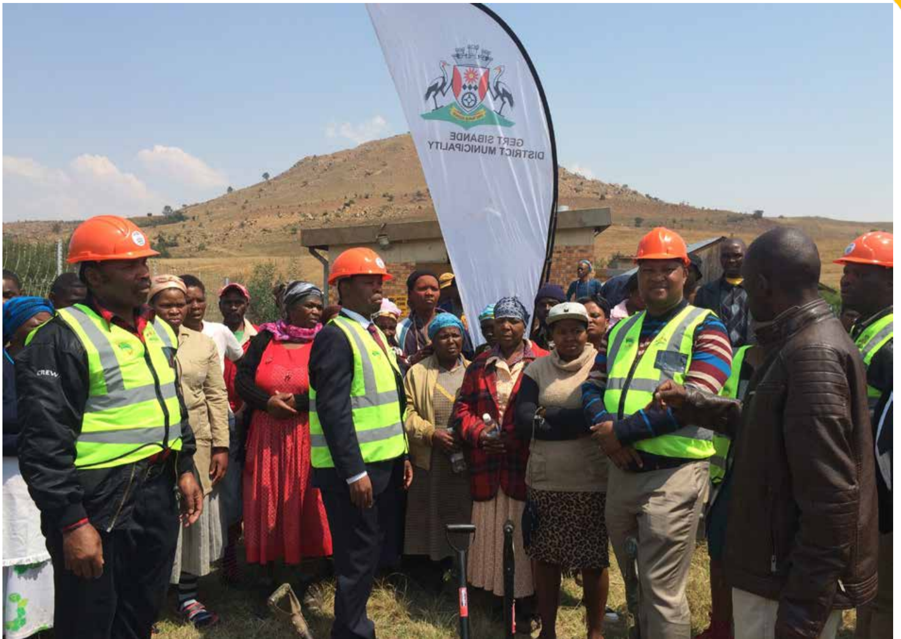
Executive Mayor of Gert Sibande District Cllr GM Chirwa, Chief Albert Luthuli Mayor Cllr DP Nkosi and District Municipal Manager during the Sod-turning of a water project at Bettysgoed.
