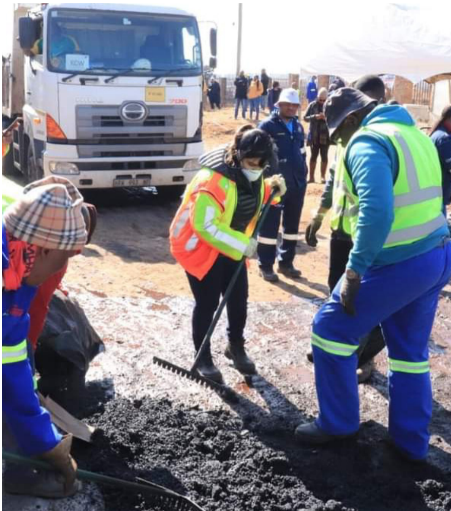
.MEC Latchminarain leading a team of officials in Balfour to fix potholes
