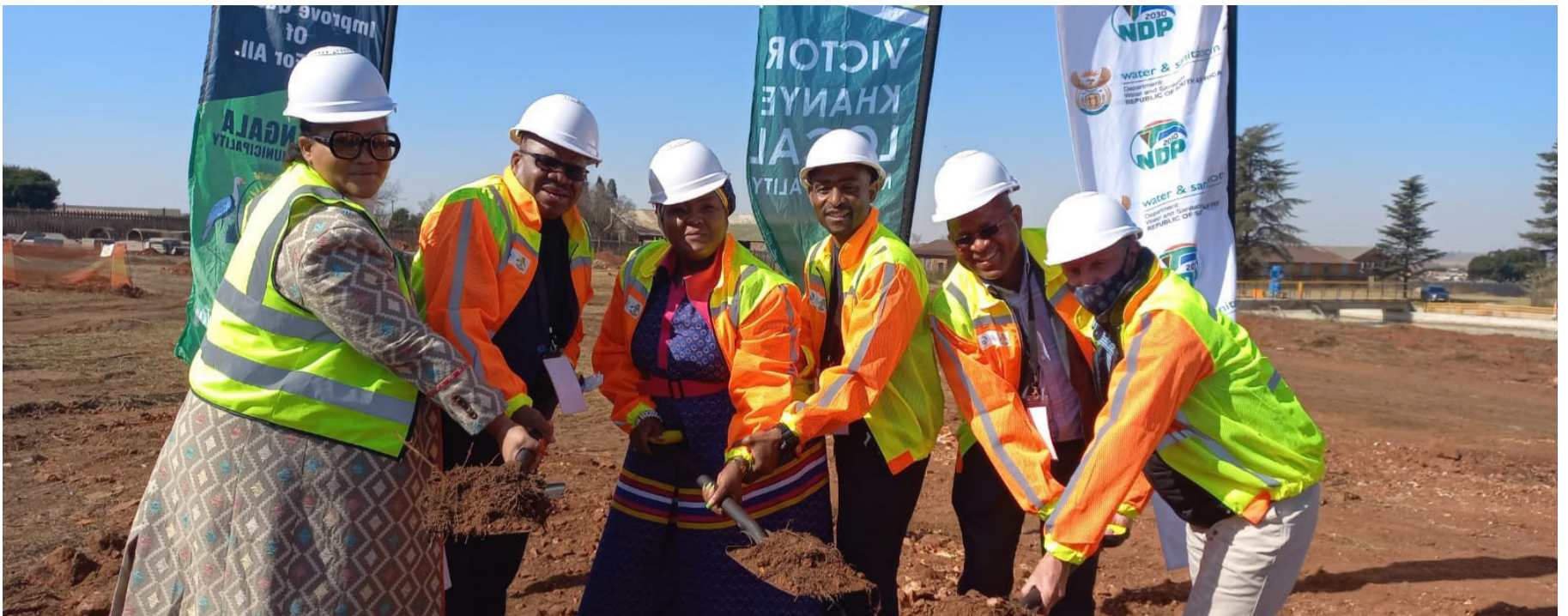
Nkangala District's Executive Mayor, Cllr. Leah Mabuza (3rd from left) leads the sod turning excursion.
